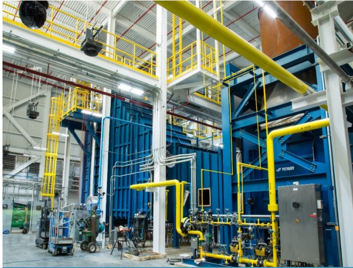
Clemson Combined Heat & Power
